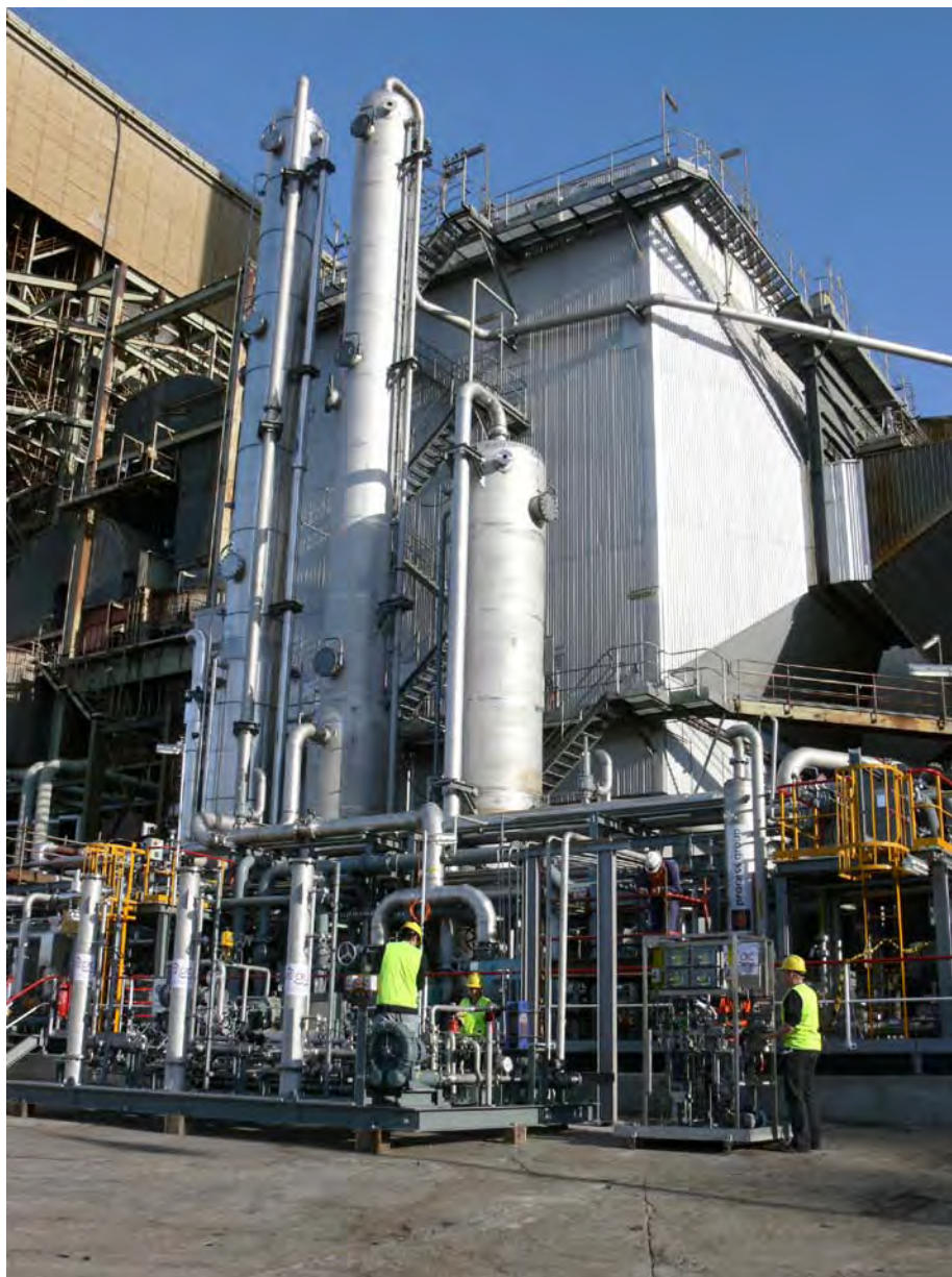
Figure 2.2: A solvent capture rig (background) retrofitted to International Power's Hazelwood coal-fired power plant in Australia to capture carbon dioxide from post-combustion flue gases (courtesy of CO2CRC).
