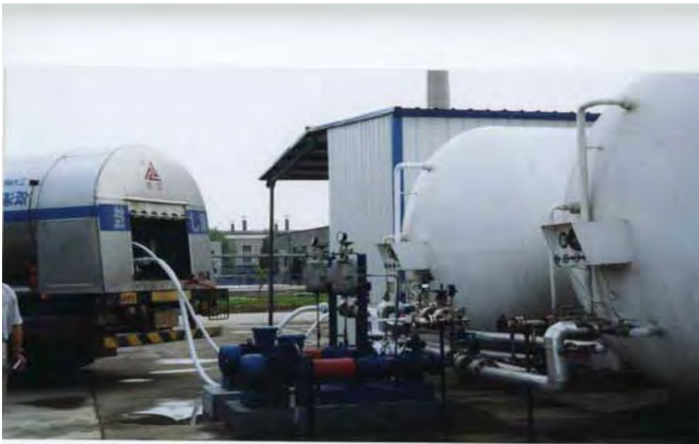
Figure 4.5: Refilling a CO 2 tanker truck.
