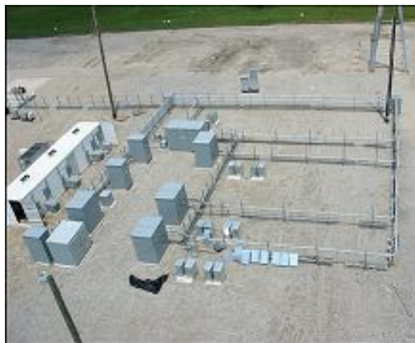
Fig.3. 1 Layout micro-grid test platforms in Dolan Technology Center
