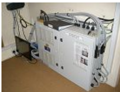
Fig.8. 16 The power switchgear and control equipment.
