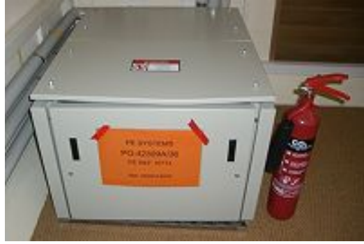
Fig.8. 18 The battery system for the “ecohome”.
