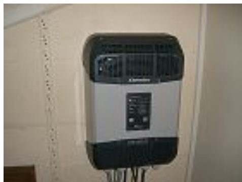
Fig.8. 17 The combined inverter and charger unit.
