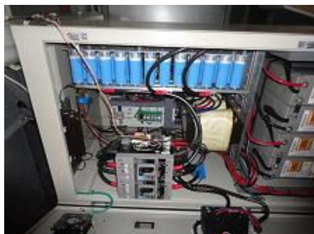
Fig.8. 6 Project Edison, the AC-DC power converter and control systems.
