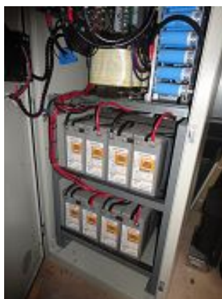
Fig.8. 7 Project Edison, the battery storage.
