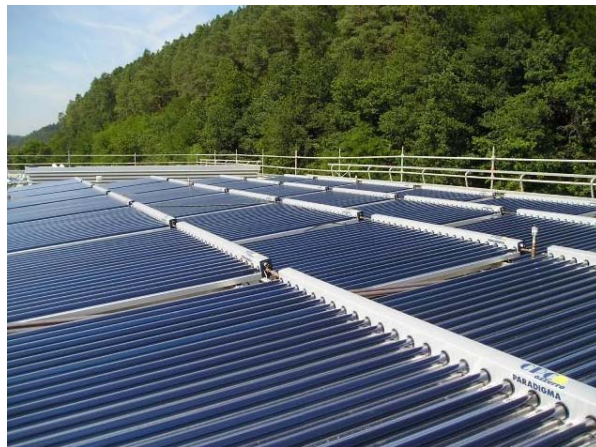
Figure 2-6: Solar Industrial Process Heat Installation using Evacuated Tube Collectors
