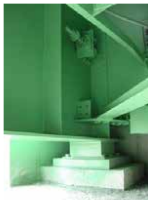
Photo 2. High Damping Rubber (Shihwei Bridge)
