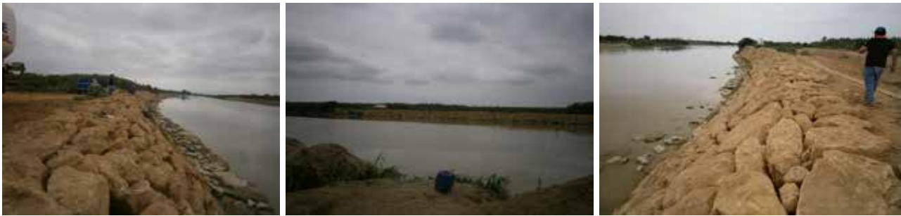
Photo. Rock casting work in the District of Tumbes protects the slope from erosion and scouring.
