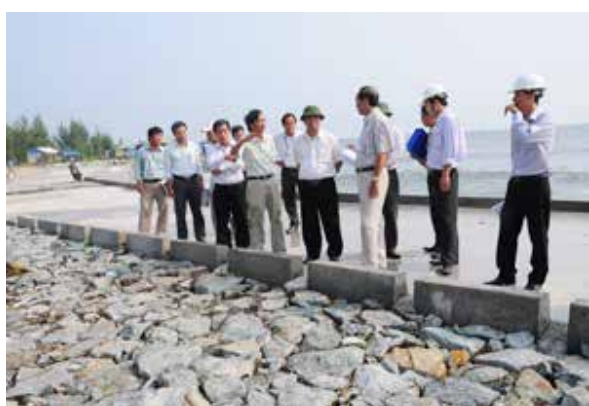
(c) The dike under construction. The PMU and provincial authority are inspecting the work.
