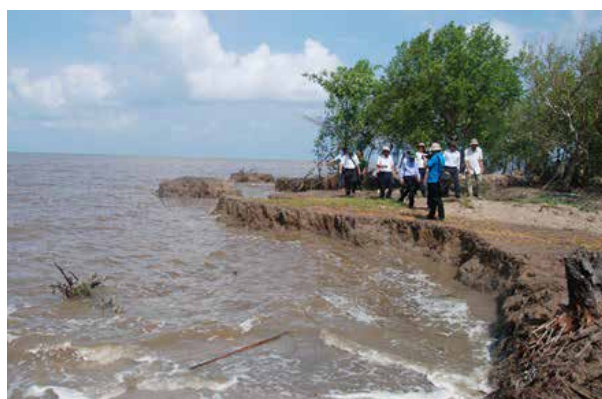
Photo 1. Landslide at West sea dike, Ca Mau province, southern Viet Nam
