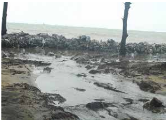
(a) Dike damaged by the storm
