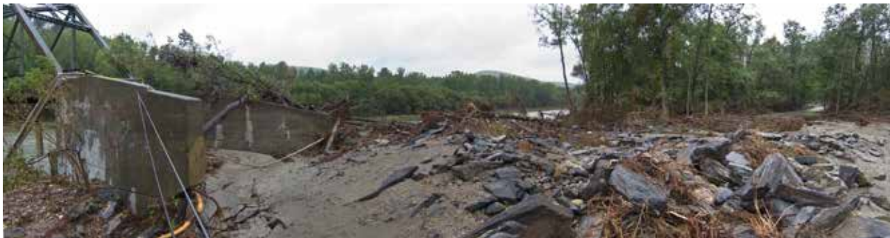
Photo: Damage caused by flood waters from Tropical Storm Irene (2011-08-28) on the Ottauquechee River in Royalton, Vermont, which scoured the approach to the bridge on the northern shore of the river, as of 2011-09-07 Source: courtesy of Wikimedia Commons
