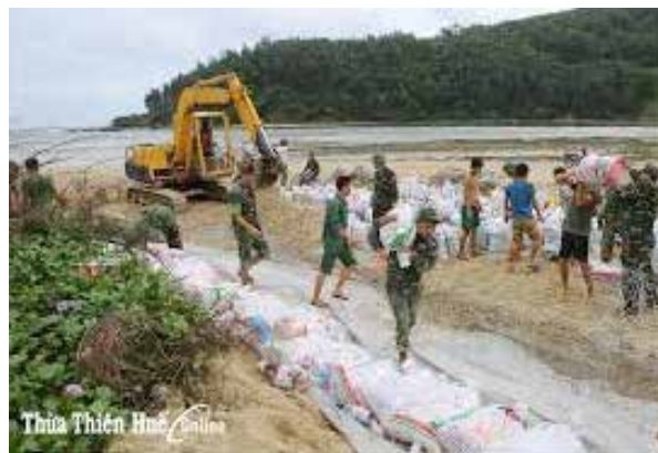
(b) Urgent and temporary repair of the road by soldiers and private citizens
