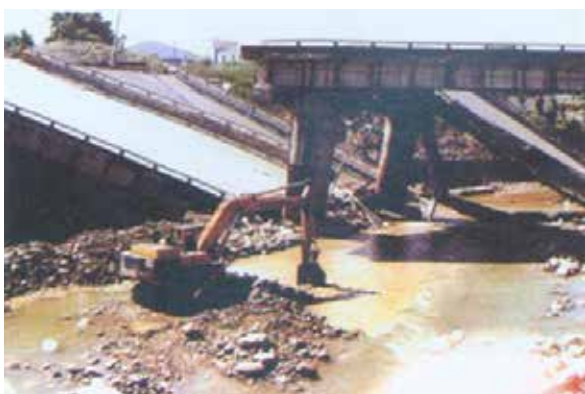
Photo 1. Damage to Shihwei Bridge due to the 921 Earthquake
