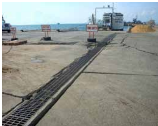
Photo. Cracks in the pier
