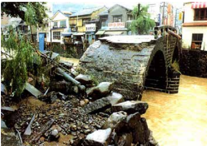
Photo 2. Damaged Megane Bridge
