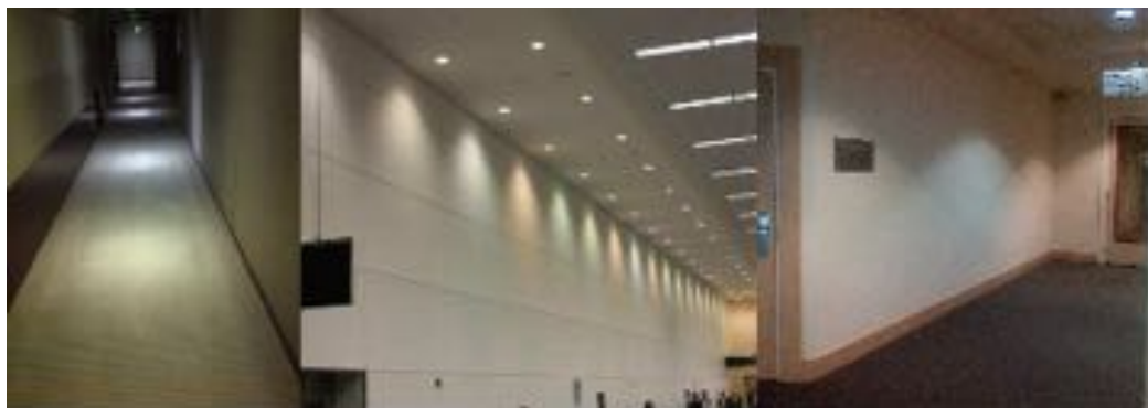
Figure 18 Colour shift of some LED lighting products
