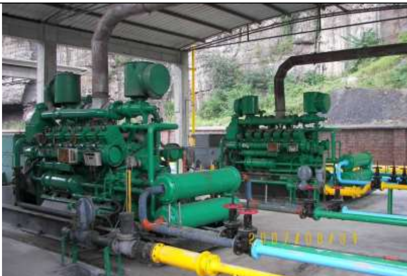
Fig.3-3 CMM power generation units
