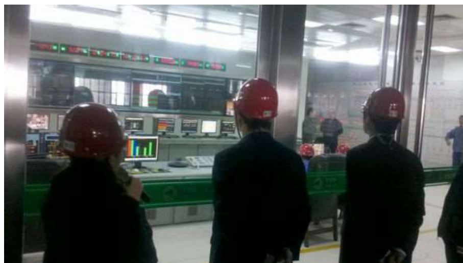
Fig.2-8 Tashan Power Co., Ltd.
