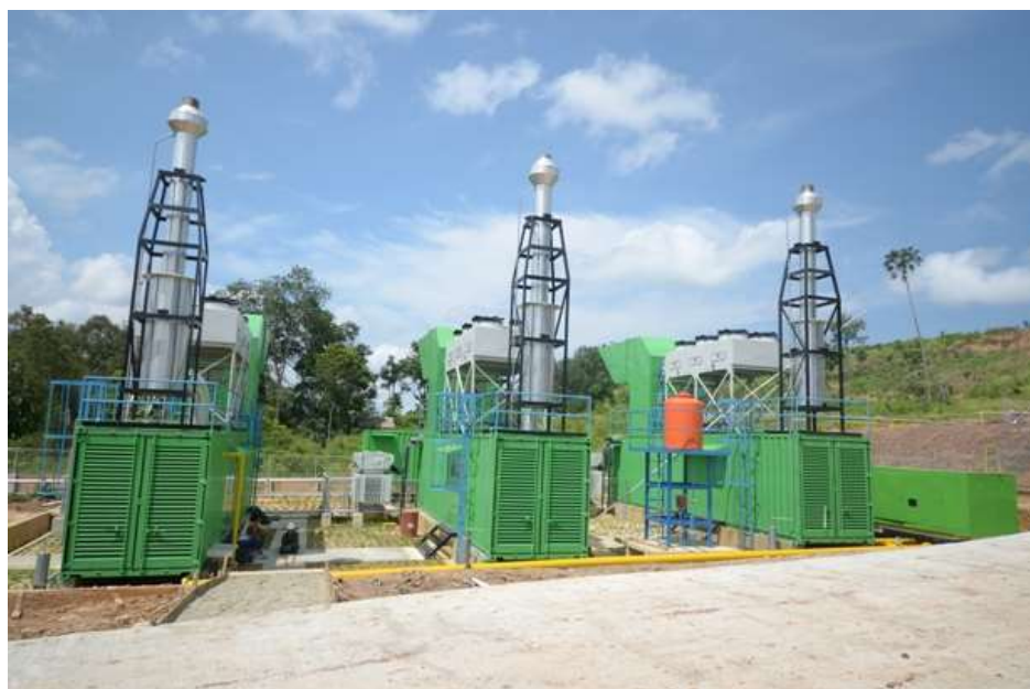
Fig.2-19 VICO CBM power generation project
