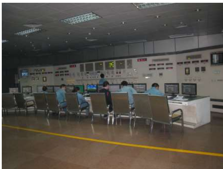
Fig.24 Monitoring room of the wastewater treatment plant in Yaoqiao Coal Mine
