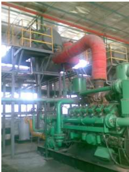
Fig.2-10 CMM power plant in No.4 Coal Mine of Pingmei Shenma Group
