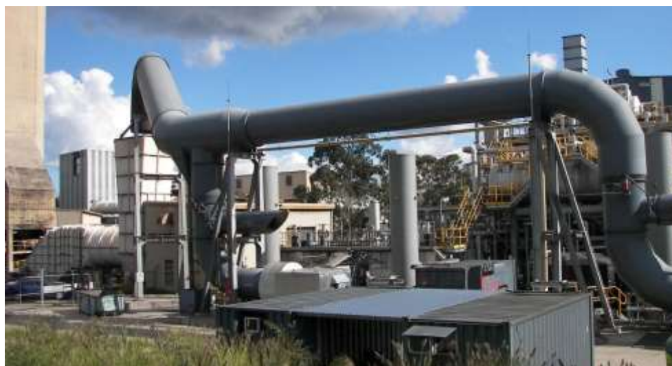
Fig.3-4 VAM power generation project in Australia
