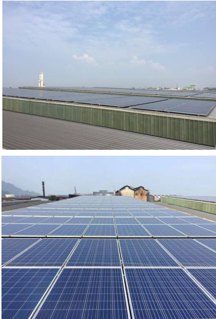
Figure 5.2 The rooftop PV system at RK South Asia Sdn Bhd factory
