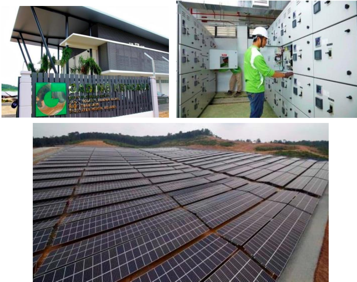
Figure 3. 14 Solar Farm Case Study 1, Malaysia
