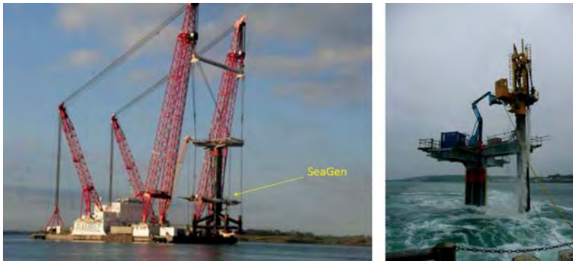
Figure 13. Crane Barge Rambiz arriving in Strangford Lough in late March 2008 to commence the installation of SeaGen (left). Drilling and grouting operations, carried out from temporary work platform (right)
