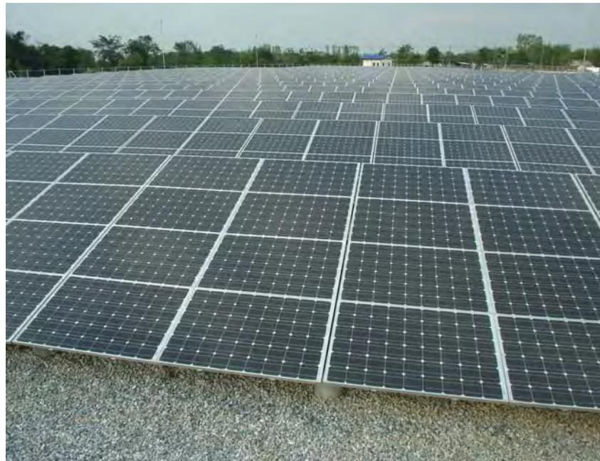
FIGURE 9-8 : A picture of Solar Farm
