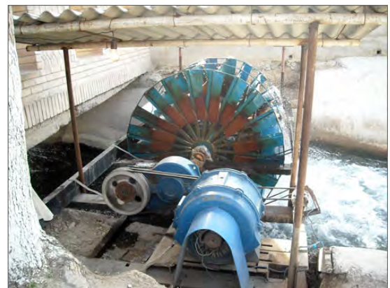
FIGURE 9-18 : Water wheel of small hydroelectric power plants
