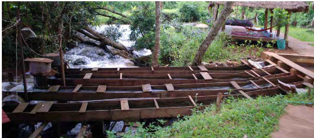
FIGURE 9-23 : Channel for water flow to the turbines
