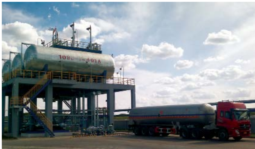
Figure 8-7 Outdoor Scene of Shenhua 100,000-ton/year CCS project
