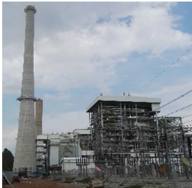
Figure 5-8 100MW CFB with Pure Combustion Biomass (Biomass Electricity Co. Ltd. in Thailand)
