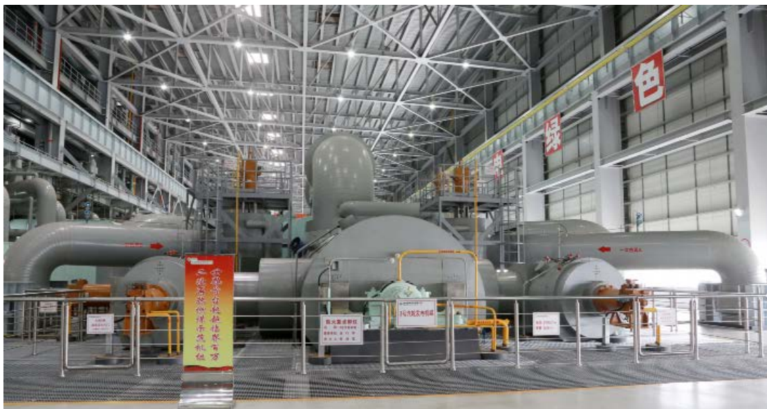
Figure 4-6 Taizhou Phase II Double-Reheat Steam Turbine
