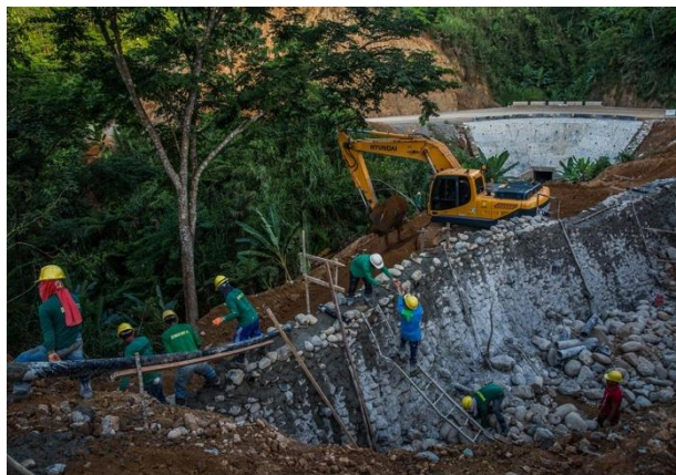
Construction of the 82km provincial road that will connect Divilacan to Ilagan city, the capital of Isabela (Photo credit: Kemal Jufri, for the New York Times)
