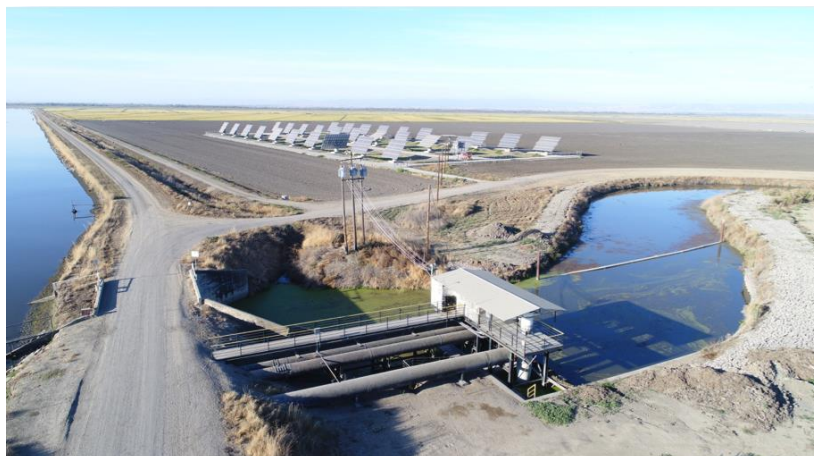
Figure 12.13 Pumping plant of water reuse, Sycamor.
