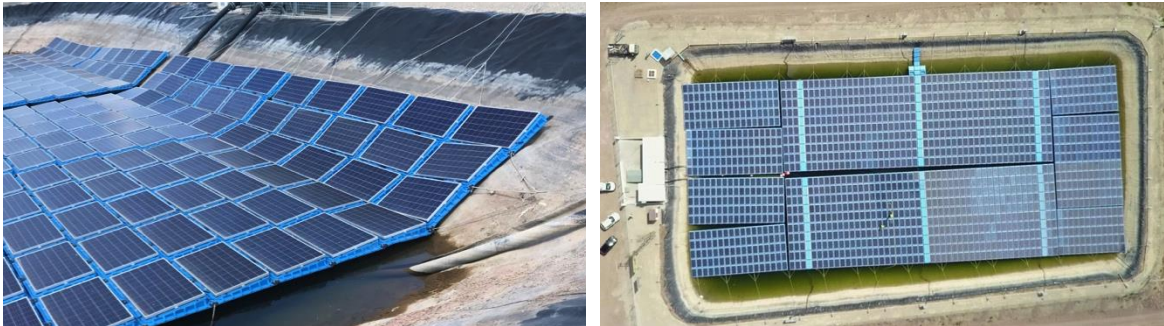
Figure 31. Floating system installed in different conditions of water reservoirs.
