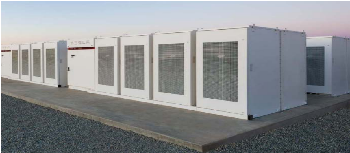
Fig. 3-6.1 Tesla 100MW Energy Storage
