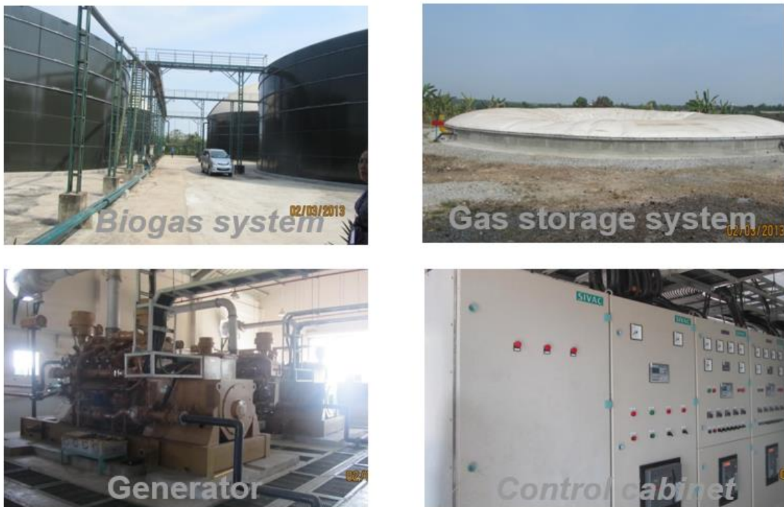
Figure 1.21: Biogas power project at the sow farm of Animal Feed JSC San Miguel
