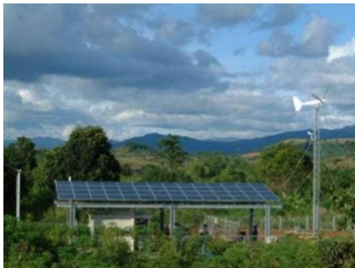
Figure 1.17: EVN's 7 kW wind-solar hybrid system in Kontum, Viet Nam
