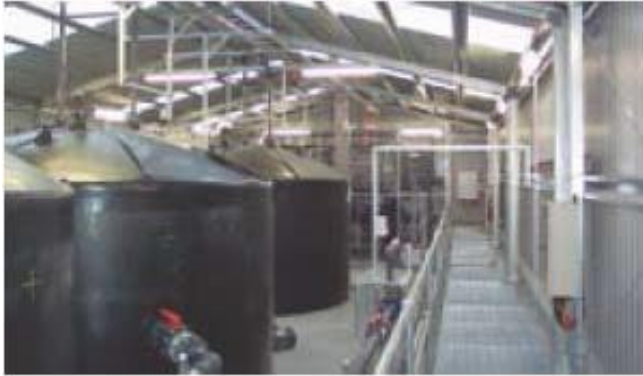
Figure 16 - Vanadium Redox Flow Battery Electrolyte Containment Vessels [117]
