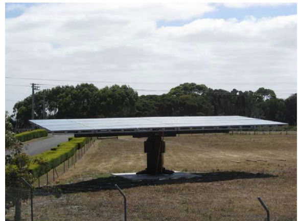
Figure 17 - Hydraulic Dual axis Tracking Solar Installation [117]
