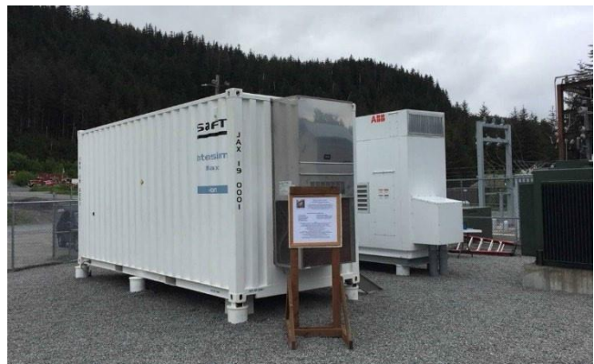
Figure 7 - Containerised BESS - Cordova, Alaska [163]
