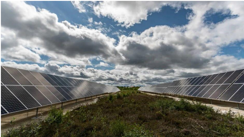
Figure 42 - Old Crow Utility-scale Solar PV system [180]
