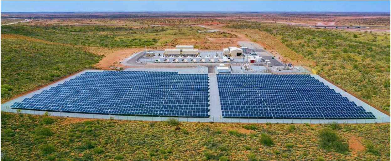
Figure 4 - Utility-scale solar and energy storage - Onslow, Western Australia [3]
