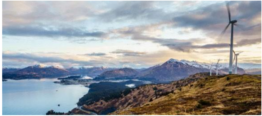
Figure 31 - Kodiak Island Wind Farm [174]
