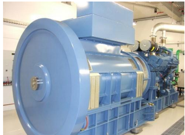
Figure 6 - Flywheel - King Island, Tasmania [162]
