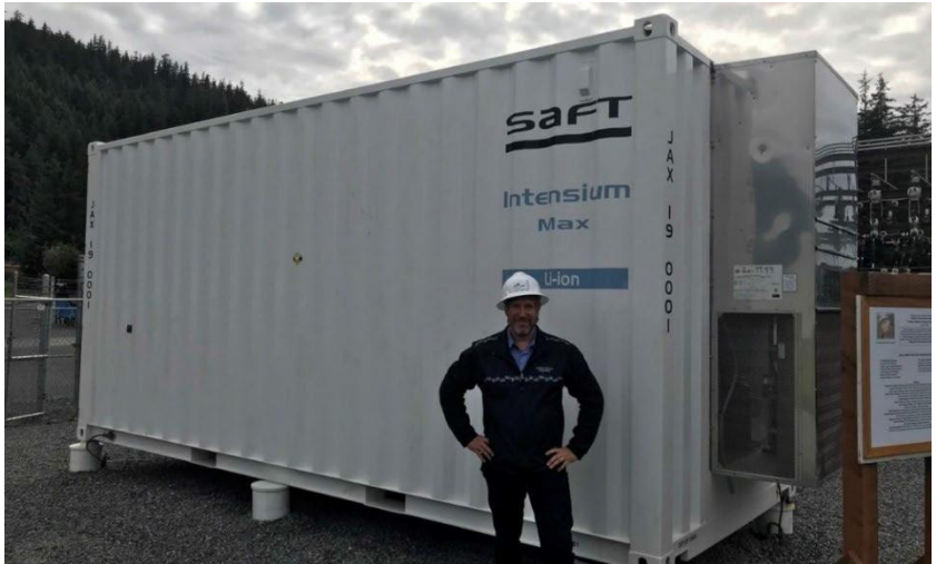
Figure 36 - Cordova SAFT Lithium-ion Battery Storage System [176]
