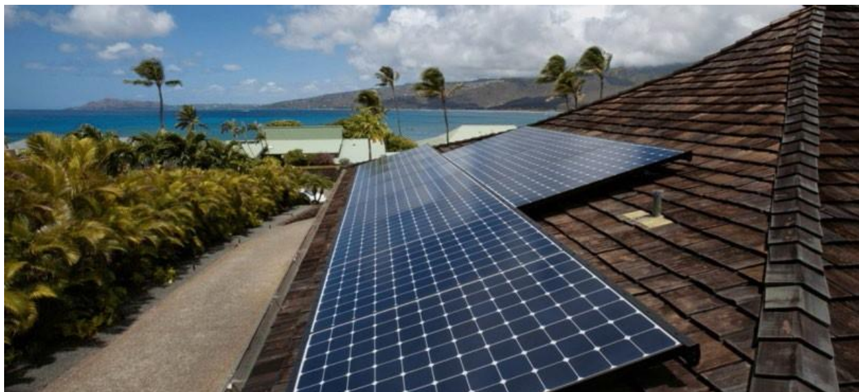
Figure 40 - Hawaii Rooftop Solar [43]
