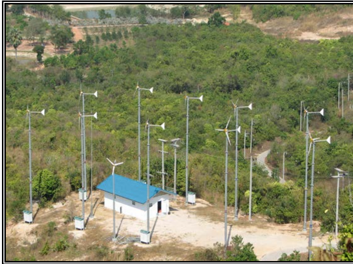
Figure 6: The First Thailand Wind Farm 200 kW at Lan Island
