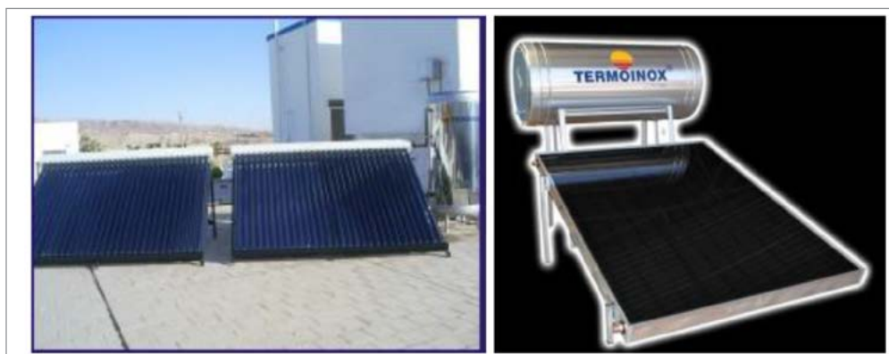
Figure 7-18: Evacuated Tube Collectors and Flat-plate Collectors Common in Peru
