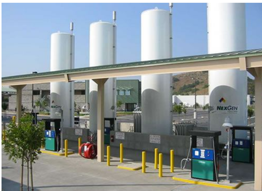
Figure 3.5: Depot Refuelling with 6 LNG Dispensers and 3 LCNG Dispensers
