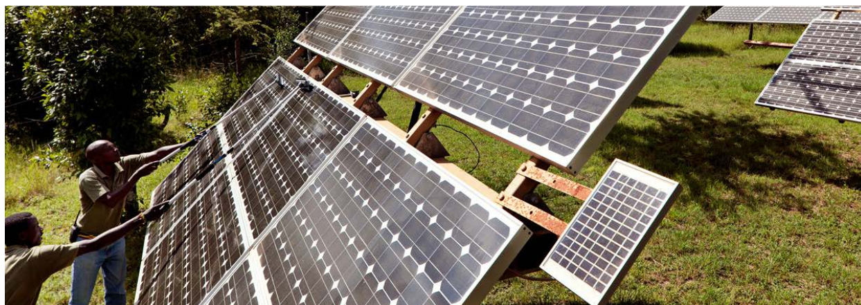
PV Panels in Senegalese Solar PV Project
