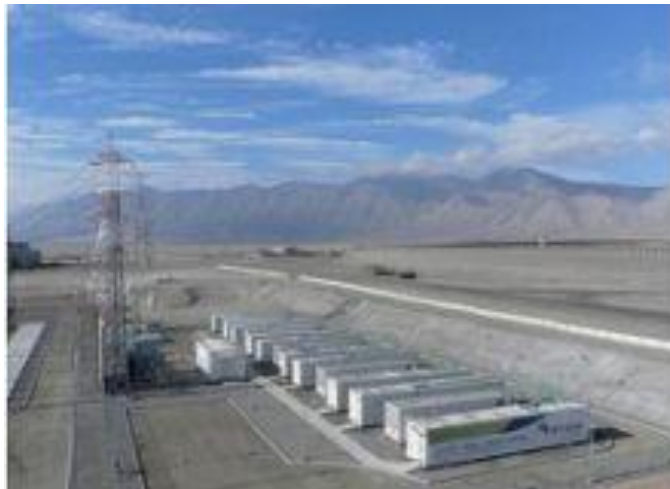
Figure 3- 10 Battery Energy Storage System (BESS)
