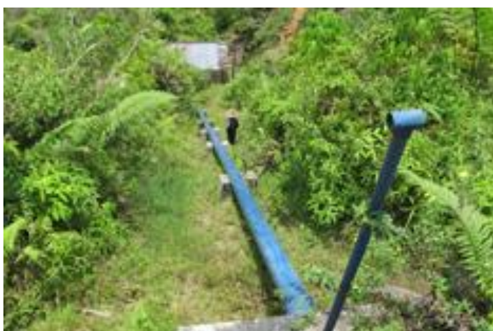
The penstock and powerhouse of the 11 kW hydro plant at Palanggaran. Source: Ashden Website
