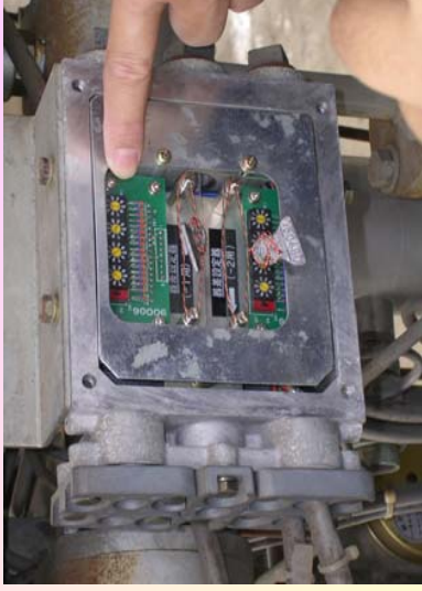
Lead sealing the flow regulator of LPG flow meter
