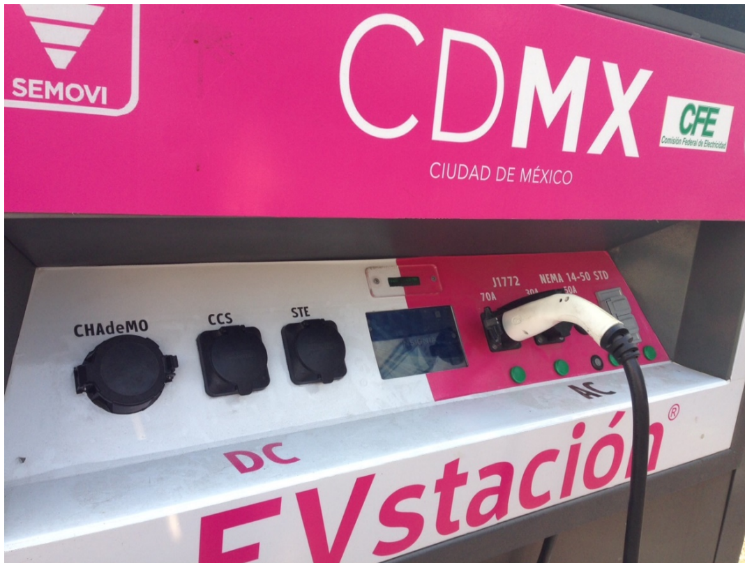
Figure 2.5 - EV charging station in Mexico City with outlets for different charging standards
