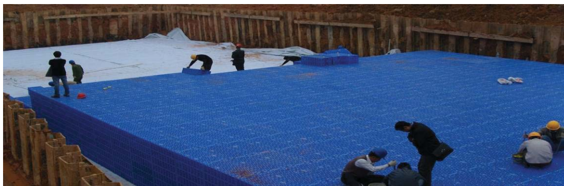
Fig. 4-12 Rainwater collecting system in construction
