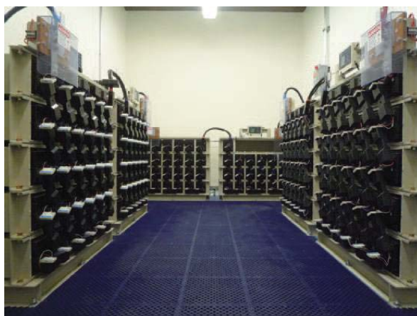
Fig. 3-4 Smart grid energy storage system in New Mexico, USA
