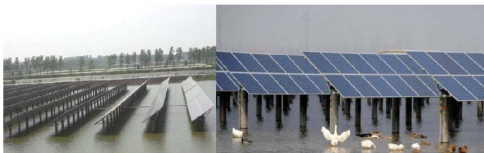
Fig. 2-9 Photovoltaic system located on fishpond
