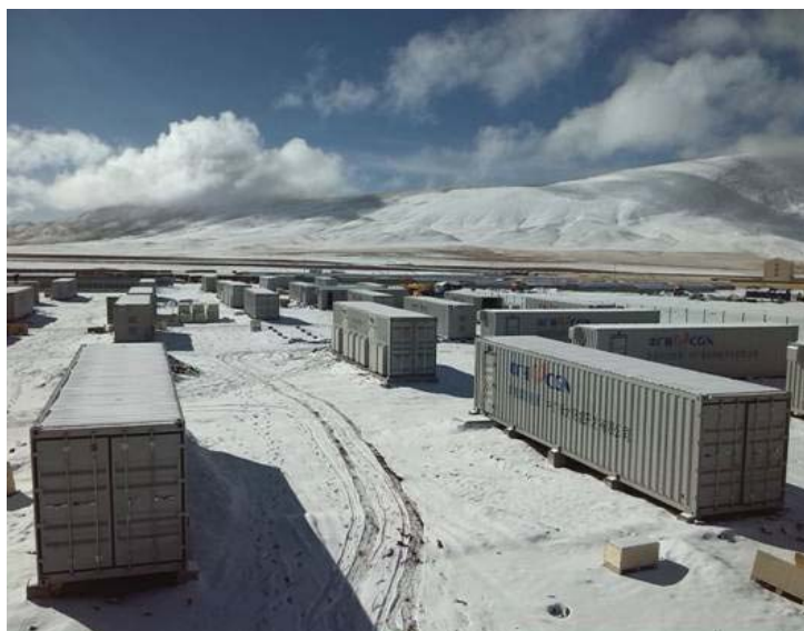
Fig. 3-8 Photovoltaic Energy Storage Power Station in CGNPC
