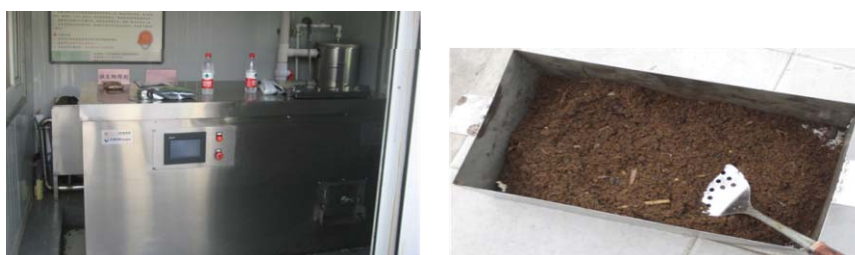
Fig. 4-17 Kitchen waste treatment system
