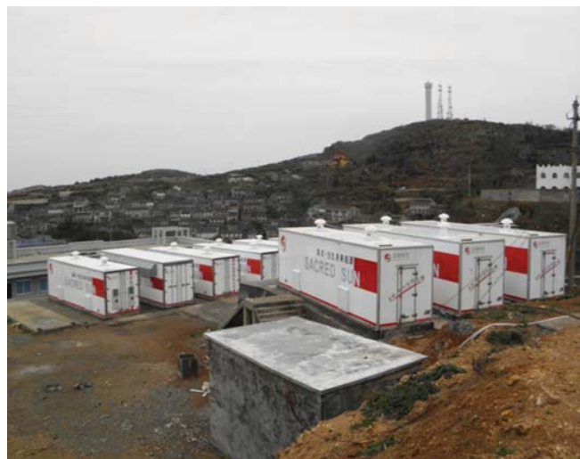
Fig. 3-11 1.274MW Micro-grid Power Station energy storage system
