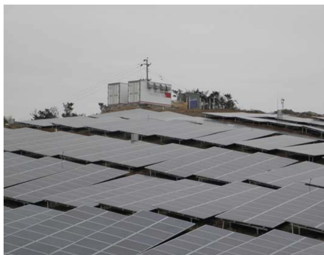
Fig. 3-10 1.274MW Photovoltaic-battery-diesel Micro-grid Power Station
