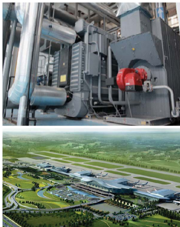
Fig. 2-18 Changsha Huanghua international airport terminal 2 CCHP Project
