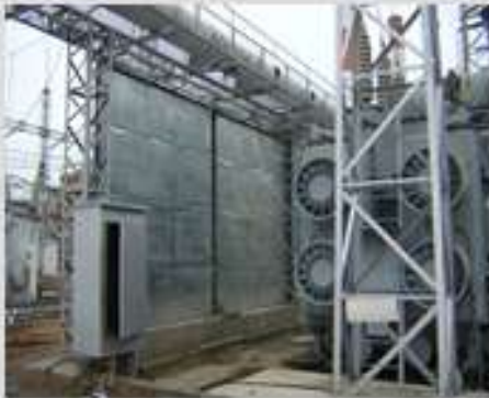
MEI acoustic screens to reduce the noise of transformers
