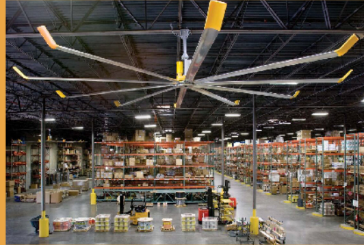
▲ Big Ass Fans' HVLS fan was applied in a warehouse, improving air circulation and energy efficiency.
