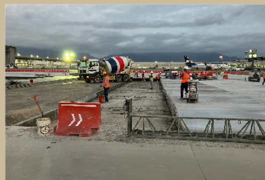
▲ Cemex's Vertua lower-carbon concrete helped to build Terminal 2 at Puerto Vallarta International Airport in Mexico.
