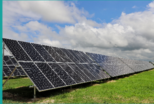
▲ Complex Mountain PV Power Station in Guizhou, China
