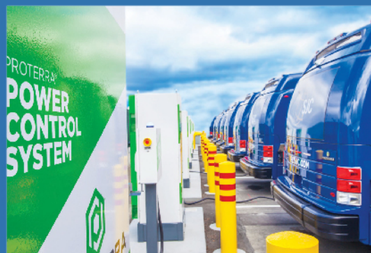
▲ Proterra's new line of fleet charging units enables charging of up to 20 transit buses simultaneously.
