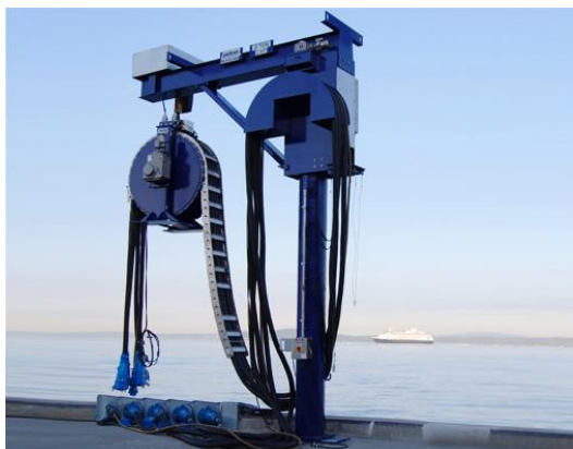
Figure 2-13: Power cable at pier
