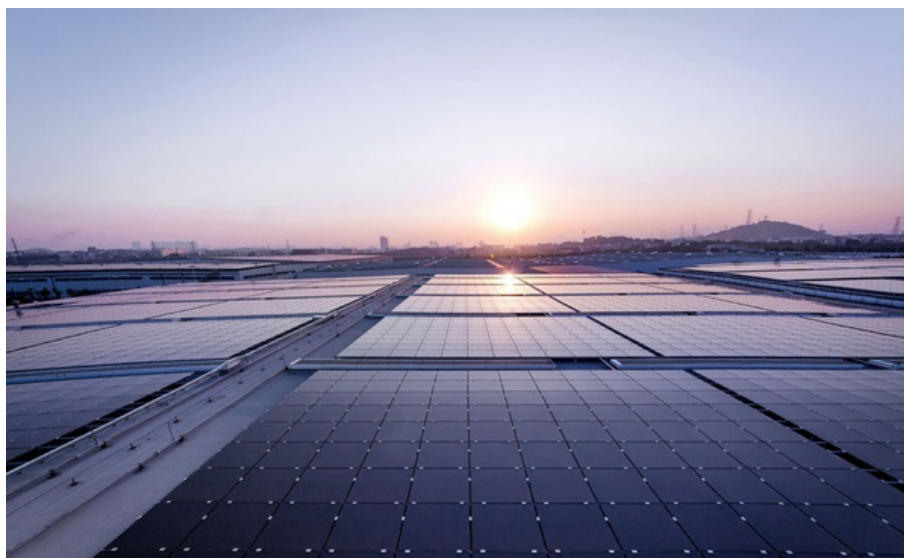
Fig. 2-3 Roofing PV system with standard PV module
