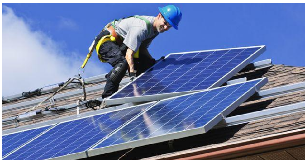
Fig. 3-12 Solar home systems in Australia
