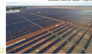
Jemalong 50MW Solar Project
