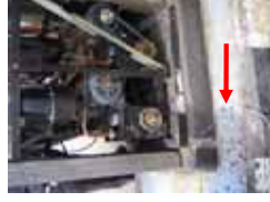
Cabling in fuel dispenser
