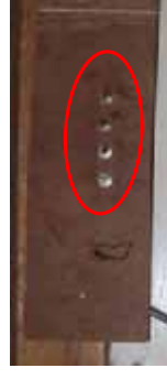
Switch On/Off in control room
