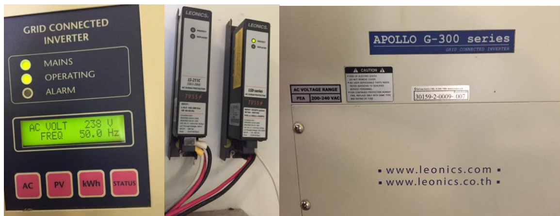
Photo 9 : Component of the smart grid PV system, Thailand
