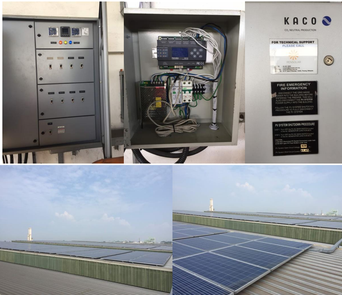
Photo 7 : Large Scale Factory Rooftop PV System, Malaysia
