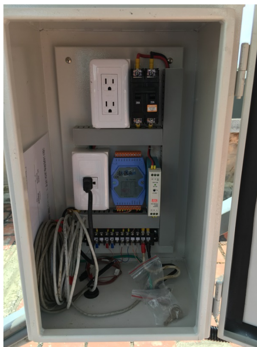
Figure 4.3.1.2 DC box of the monitoring system
