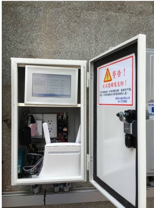
Figure 4.3.1.3 DC box of the monitoring system
