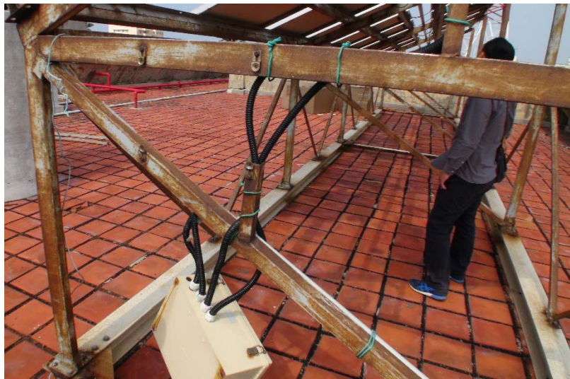
Figure 4.1.5 Corrosive phenomena on bracket
