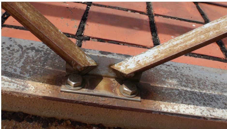
Figure 4.2.2 Stainless bracket after removing rust
