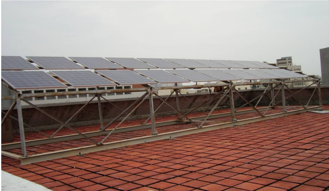
Figure 1.3.1 Overall view of the Penghu PV system
