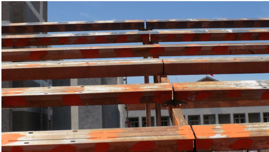
Figure 4.2.4 Surface of metal/stainless after maintenance
