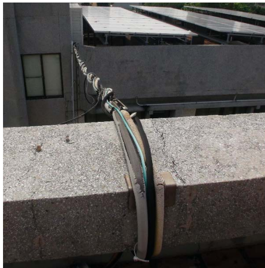
Figure 4.1.11 Anti-UV cable had aging and cracking phenomena
