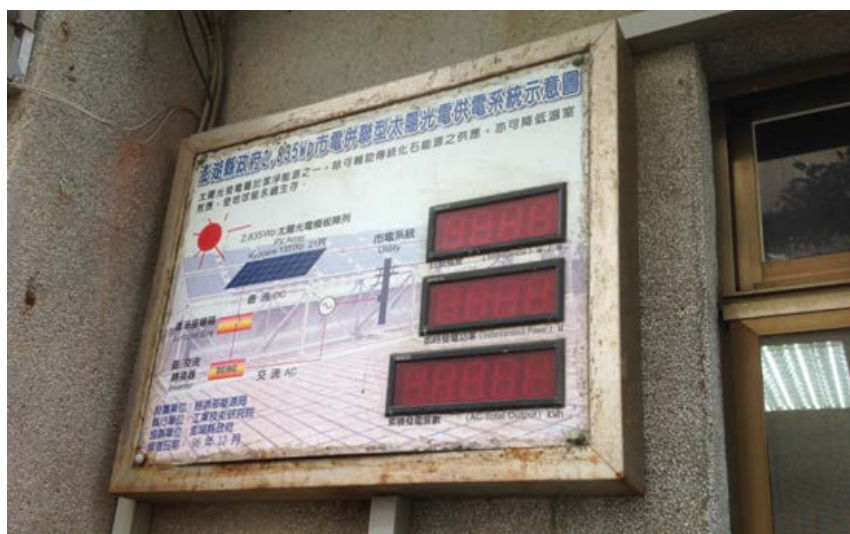
Figure 4.1.1 The monitor display of the Penghu PV system
