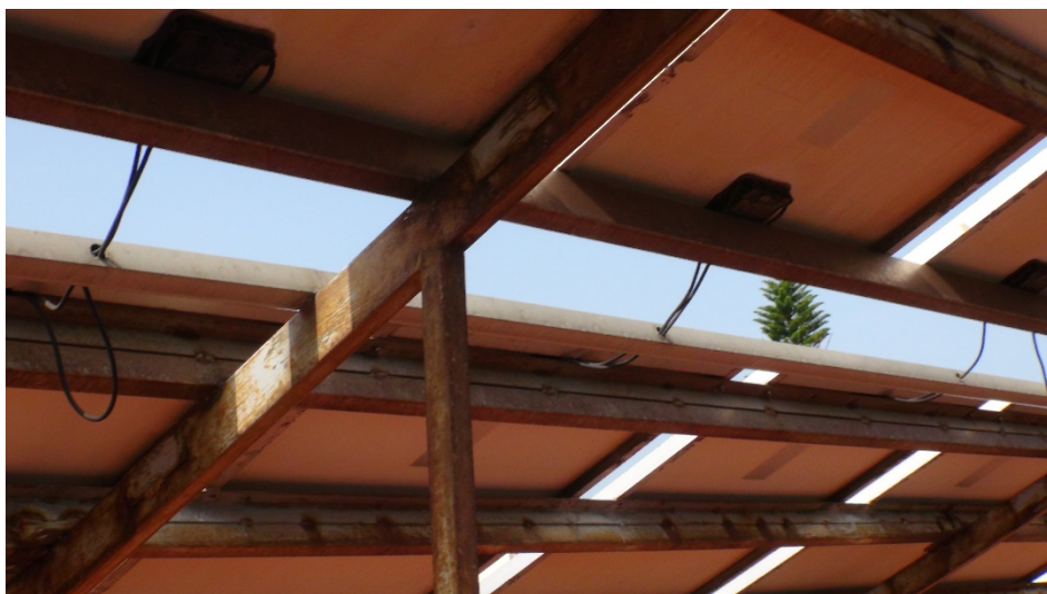
Figure 4.1.9 Corrosive phenomena on soldering point of bracket
