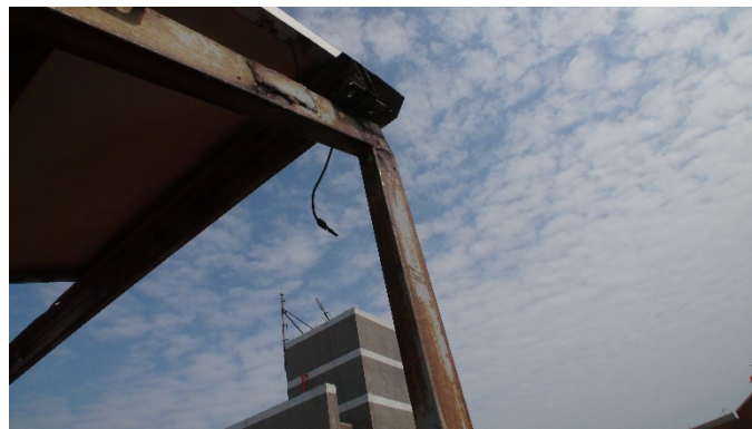
Figure 4.1.8 Corrosive phenomena on the surface of bracket
