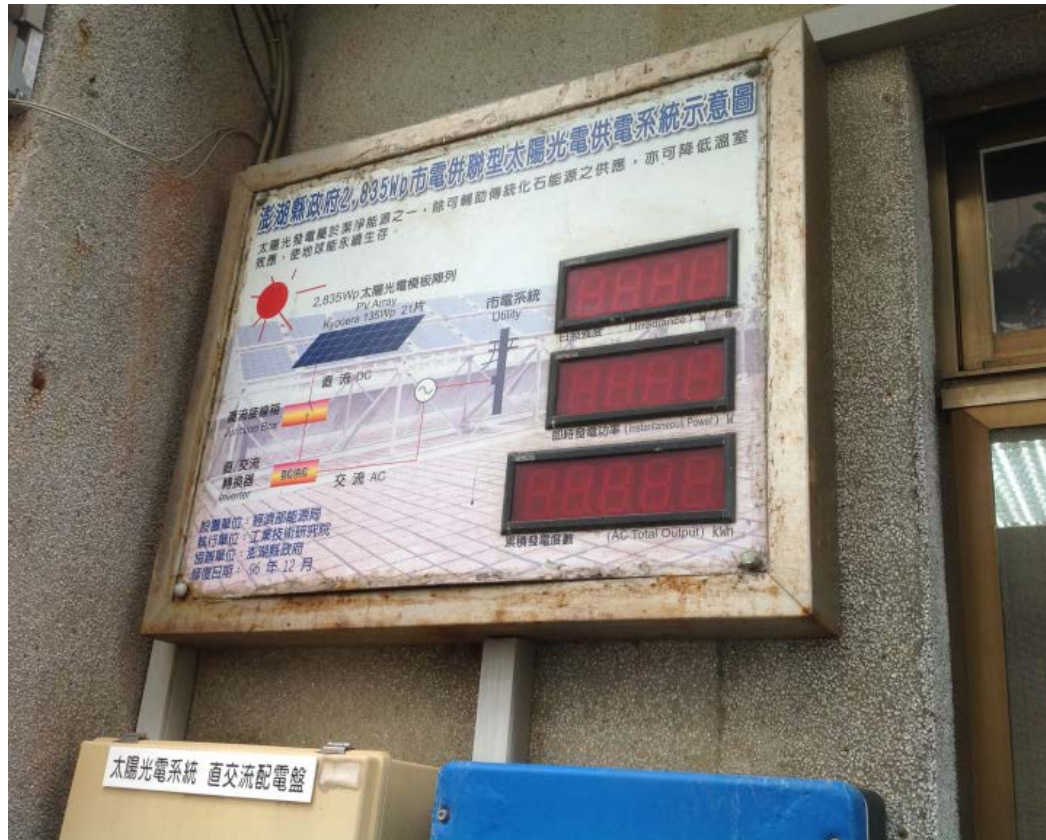
Figure 1.3.3 Monitor display of the Penghu PV system
