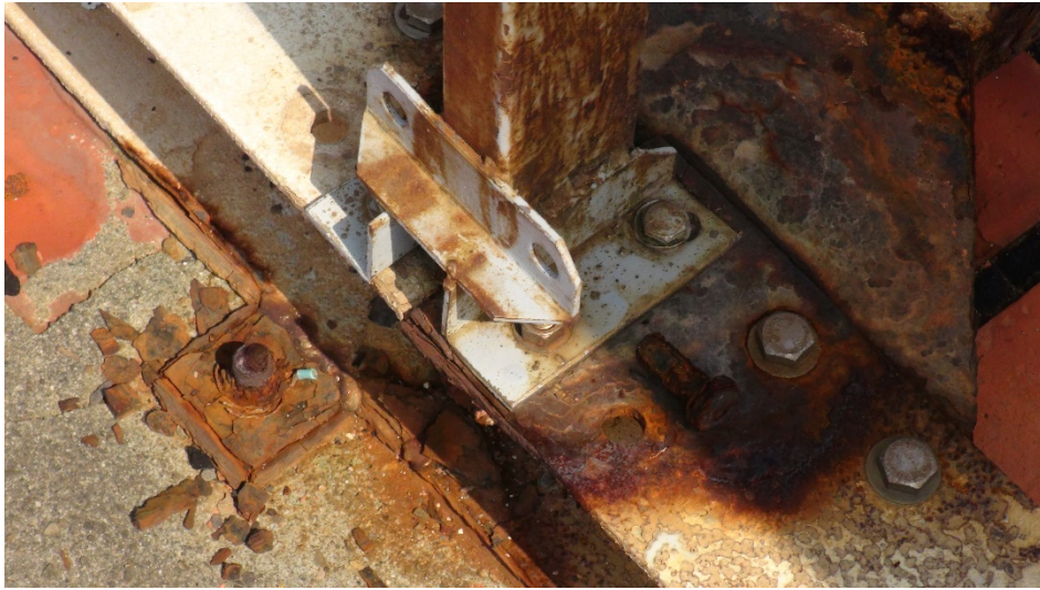
Figure 4.1.7 Contact point corrosion between bracket base, screws, nuts, and H shape stainless
