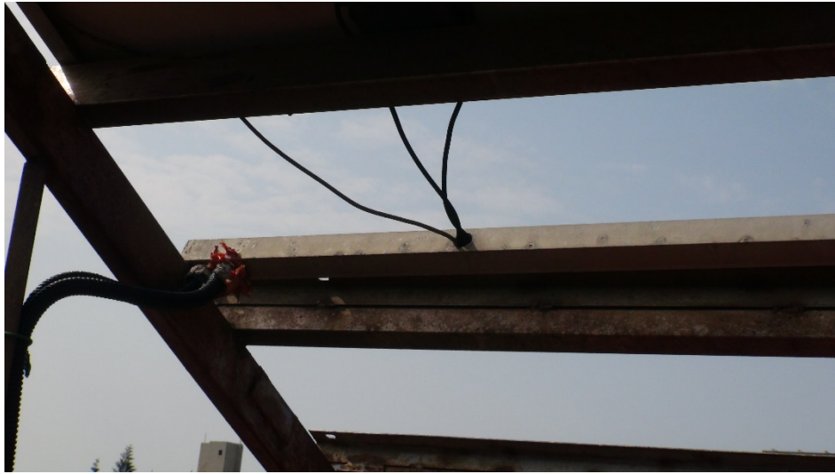
Figure 4.1.10 DC cable tray status
