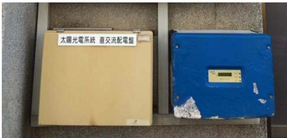
Figure 4.1.2 AC/DC power panel and inverter of the Penghu PV system
