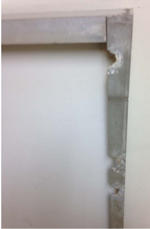
Figure 2.1.5.3.1 Potential corrosion of aluminum frame
