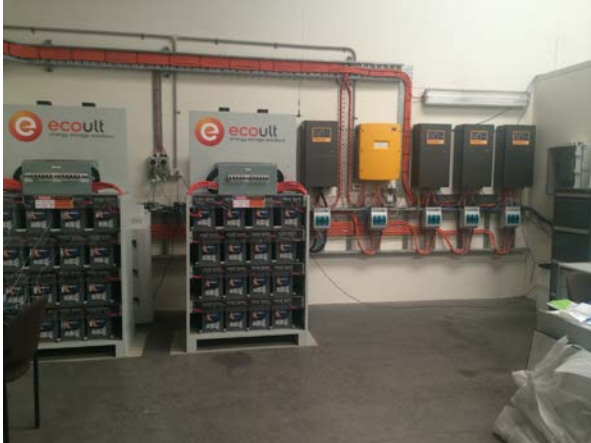
Figure 31 Energy storage unit at CSIRO Energy
