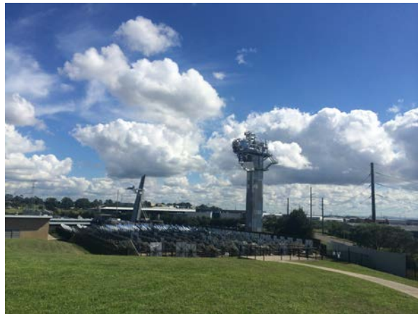
Figure 30 Microgrid system at CSIRO Energy
