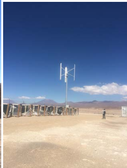
Figure 26. Small wind turbine
