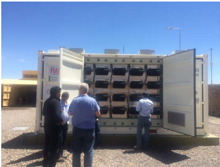
Figure 25 The battery system of the microgrid
