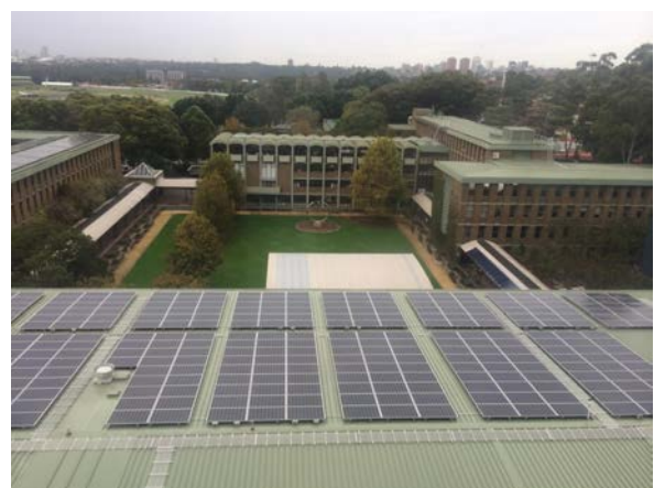
Figure 34 Solar system at UNSW
