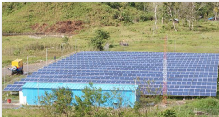
Figure 30: Oksibil Solar Power Plant
