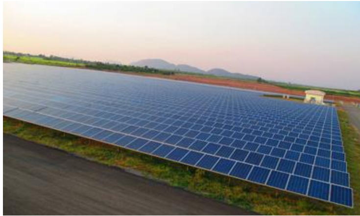
Figure 25: SSE1 PV Kanchanaburi
