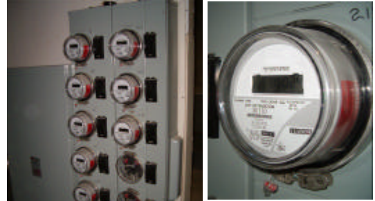
120/208v Network meters in an apartment complex
