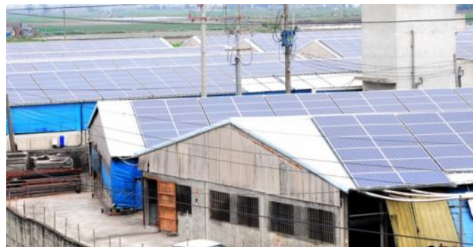
Solar panel on the swine house
